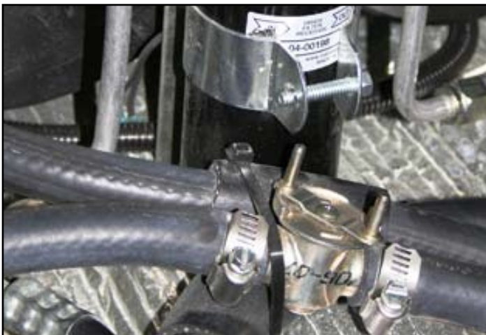
DTS manual heater control valve behind passengers seat
