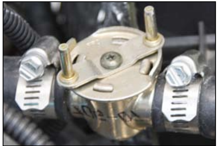
(pic. C) manual valve in on position allows hot water flow
