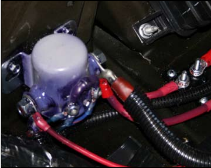
DTS power distribution module under the passenger rear seat
